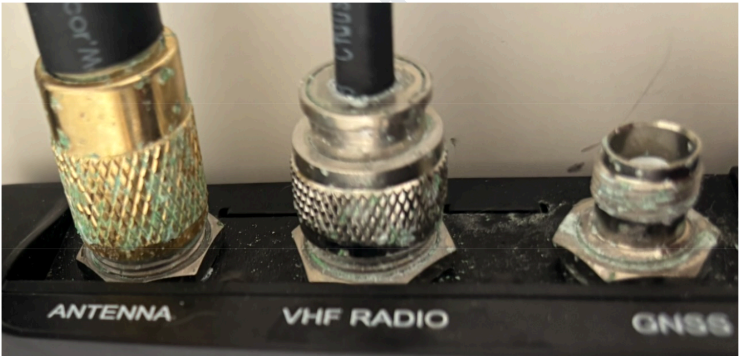
AIS connectors corroded.
